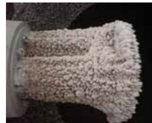
Outer unit is coated with build-up from dust.
