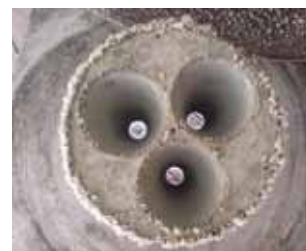
Inside the unit is clean and fully operational.
